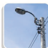
Electric Pole with Street Light
